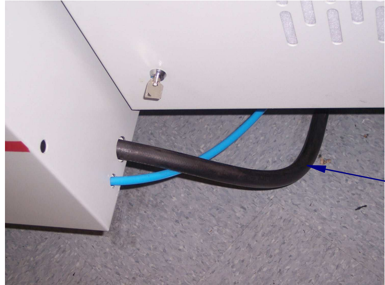
TO WASH DOWN, NOZZLE PORT
