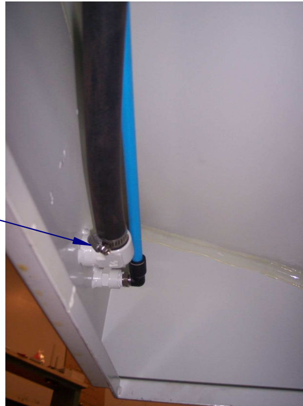
WASH DOWN PORT, INSIDE
