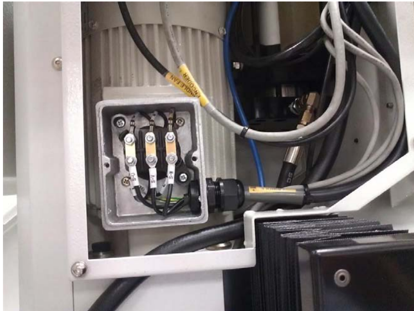
Figure 6.9b – Wiring into spindle motor – 220 volt wiring shown
