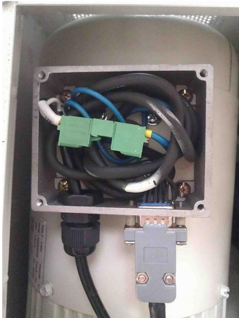
Figure 6.9c – Wiring of motor fan and encoder
