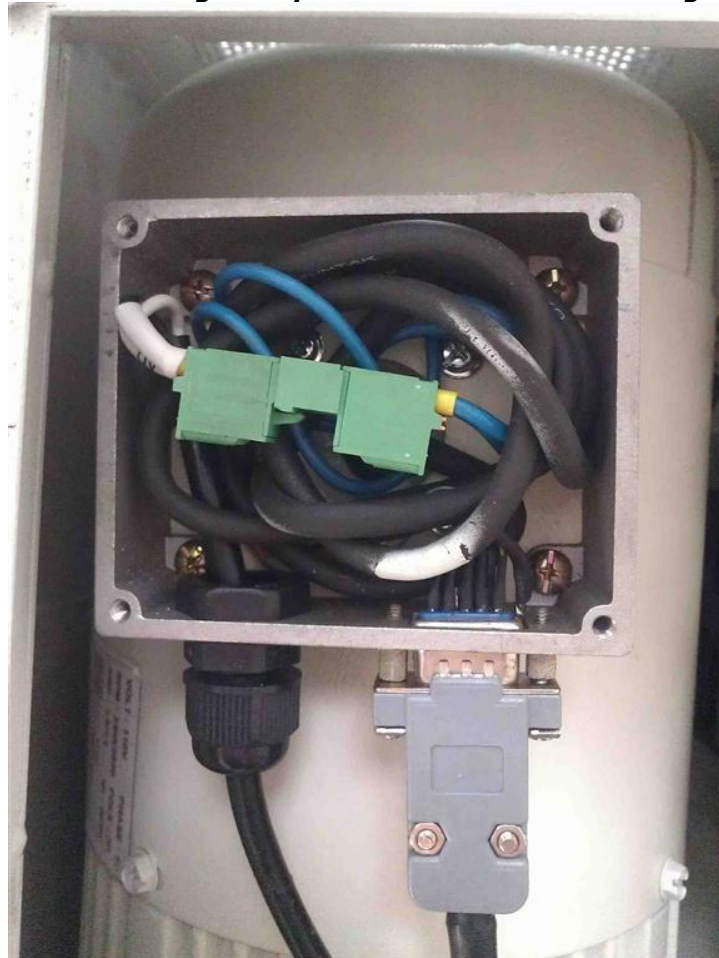
Figure 6.9c – Wiring of motor fan and encoder
