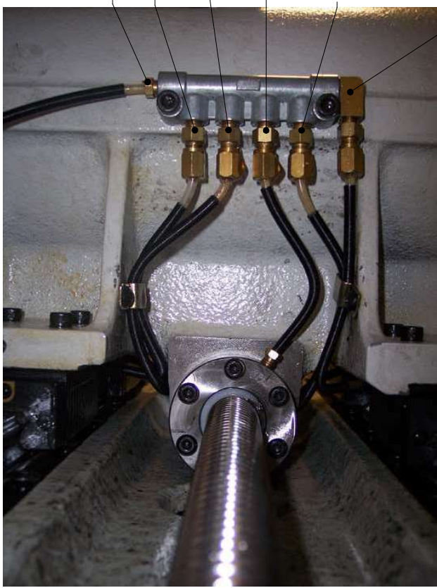
LEFT SIDE VIEW OF THE X AXIS LUBRICATION DISTRIBUTION MANIFOLD AND THE LINES TO EACH OF THE RAIL GUIDE BLOCKS AND THE BALL NUT.
